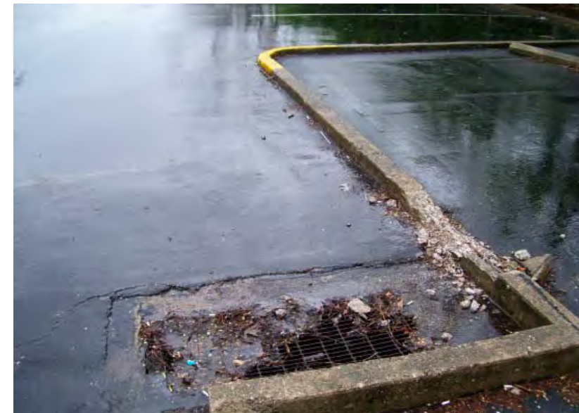
Much of Cincinnati's wet-weather flow problem is found in numerous small sources, such as this parking area inlet. As communities change for the future, the design template must actively and creatively address correction of these problems in ways that are systemically effective and cost-efficient
