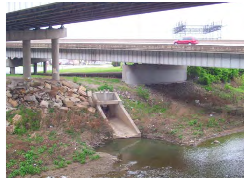
MSD has numerous assets that will be affected by the I-75 upgrade project, such as this CSO outlet near Northside/South Cumminsville.
